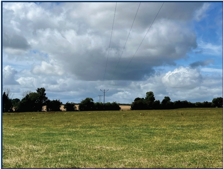
* Typical 38 kV Single pole (Shorter span technology)
