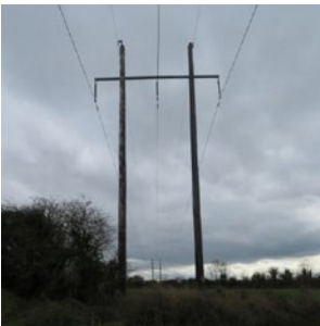
110 kV poleset with earth wire
