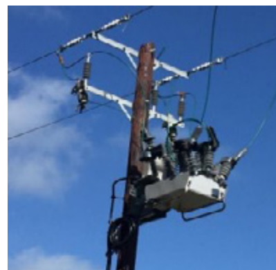
Three Phase Recloser
