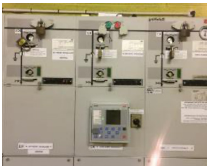
MV urban switch automation
