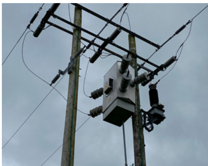
38kv remotely controlled switch
