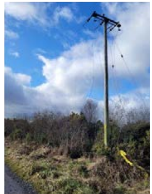
Third Party Damage causing grounded electricity line
