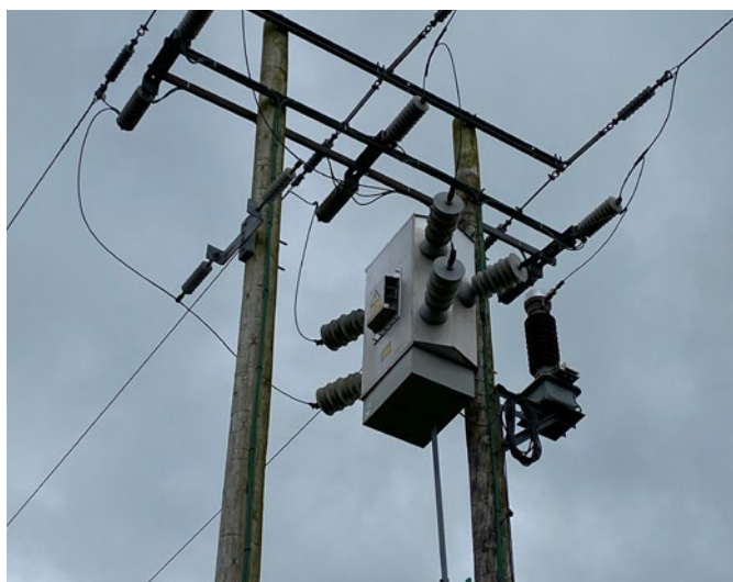
38kv remotely controlled switch
