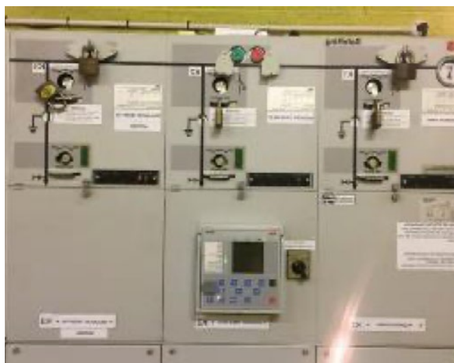
MV urban switch automation
