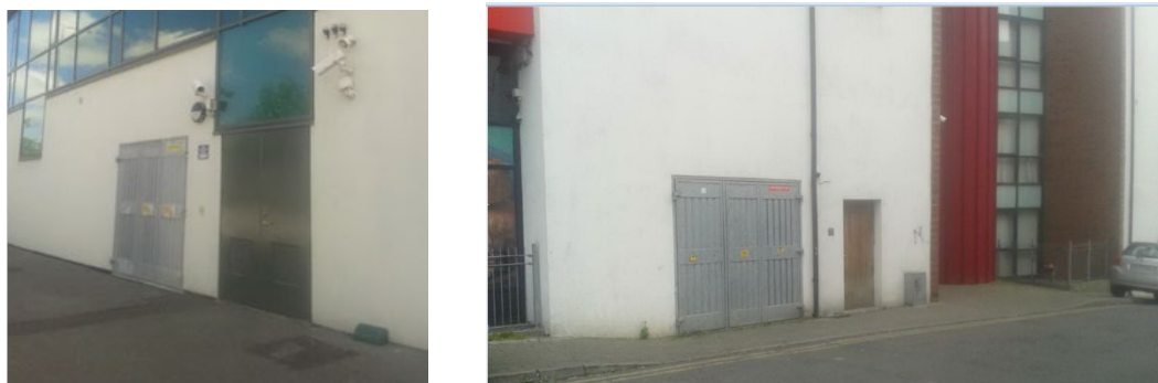
Fig. 3: MV substation incorporated into a large building development.
