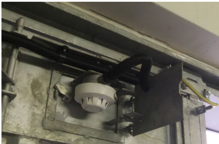
Fig. 11: Smoke detector fitted inside the hatch on substation door.
