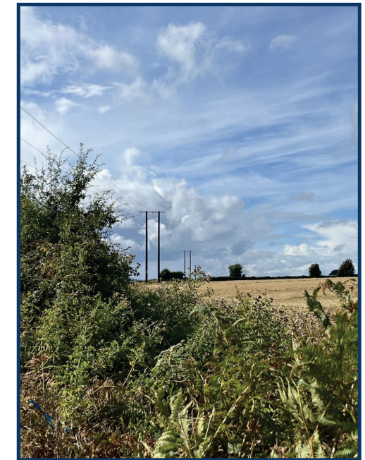
* Typical 38 kV Double Pole (longer span technology)
