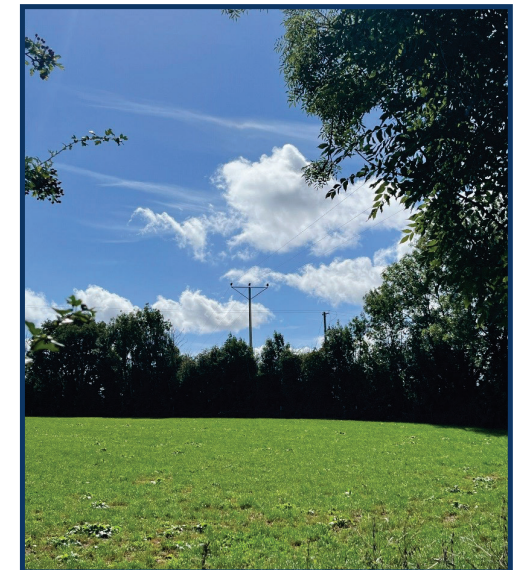
* Typical 38 kV Single pole
