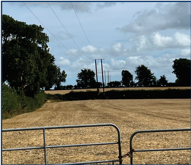
* Typical 38 kV Double Pole (longer span technology)
