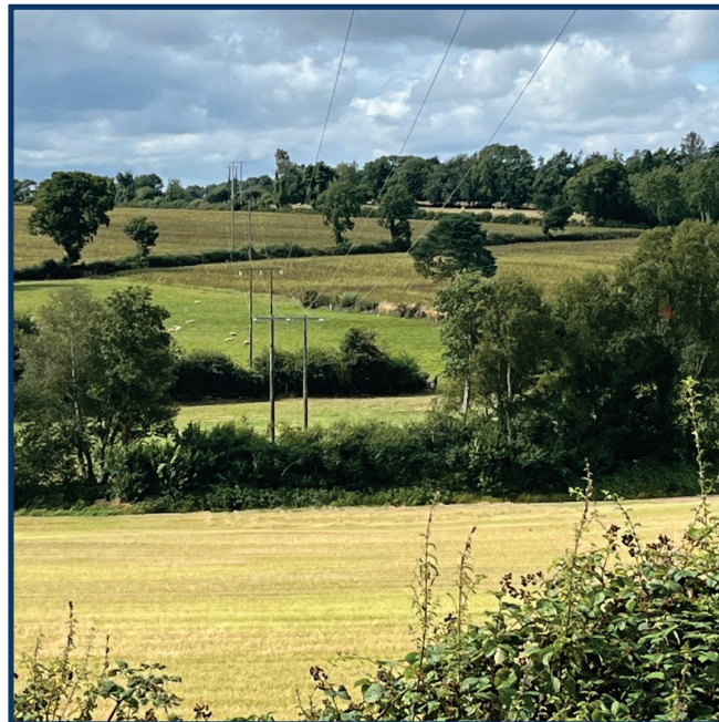
* Typical 38 kV Double Pole (longer span technology)
