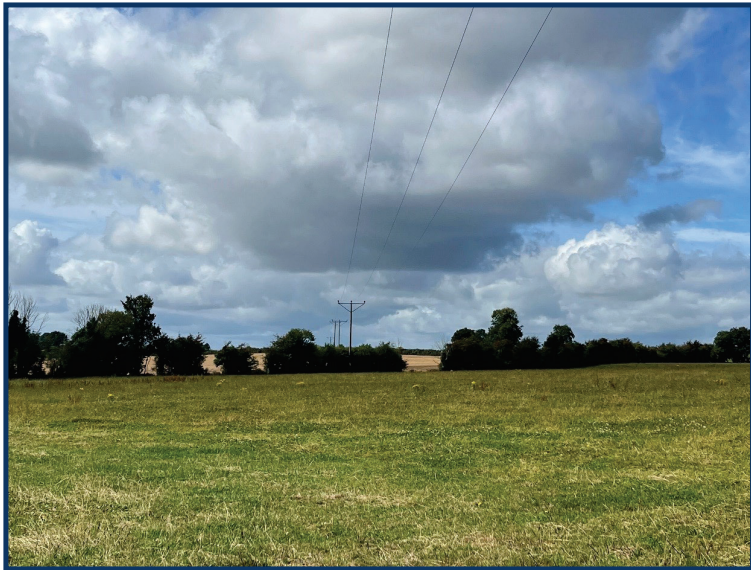
* Typical 38 kV Single pole (Shorter span technology)
